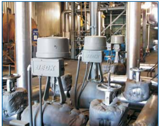
Group 14 linear drives on condensate return valves.
