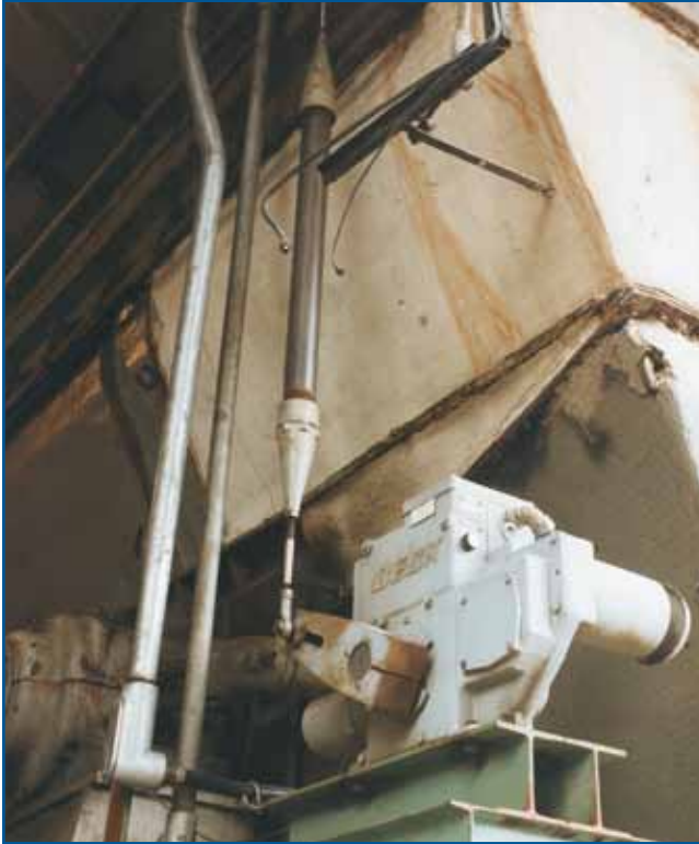
Beck replacement installed on an outdoor modulating FD fan damper. Note obsolete pneumatic lines.
