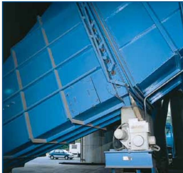
Beck drive installed on a parallel blade inlet damper.
