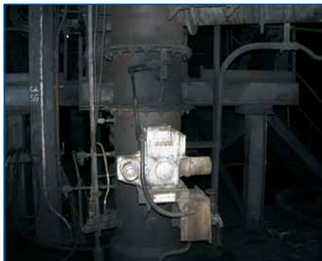
Beck drive installed on a coal mill exhaust damper.
